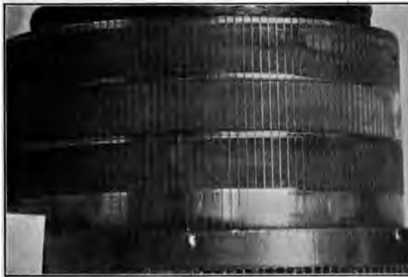
FIG 91.—Commutator showing high mica and burning of the surface on account of the attendant sparking; also ridges between brushes caused by improper brush stagger.
